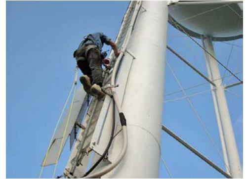
Antenna repairs require a "volunteer" to climb the tower ladder with tools in tow.
