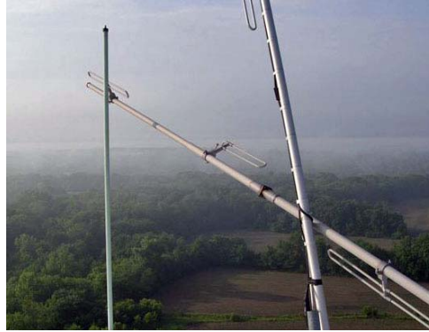
You can see for miles from the top of the Chase water tower antenna location, even with the haze. Note the abnormal antenna position.
