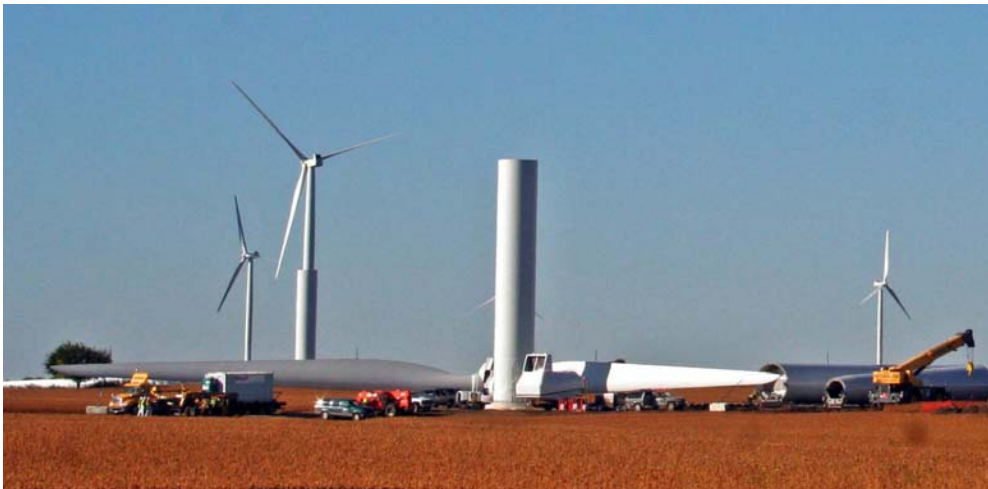
The size of the Benton Co. wind turbines is brought into perspective by noticing the trucks just to the left of the vertical structure just placed on its concrete pad. A prop is on the ground.
