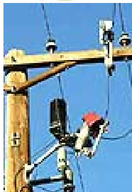
BPL system installed in Cottonwood, AZ, is being monitored by local ham club.
